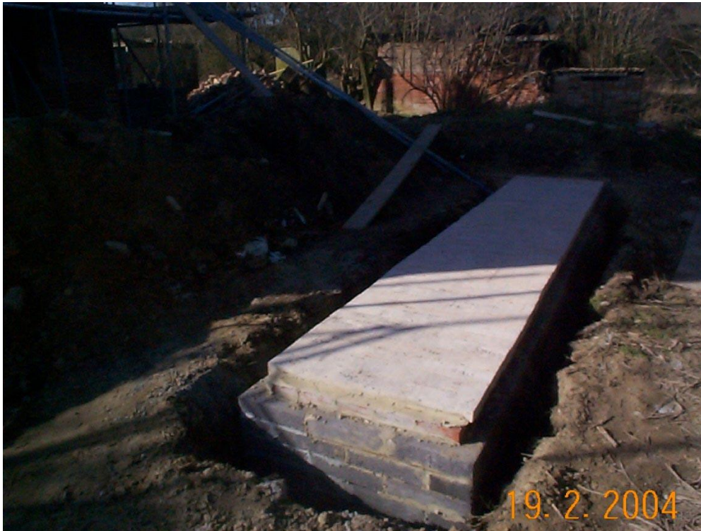
Figure 33. Part of the blockwork tunnel system connected to the maternity roost before it was covered over with earth
