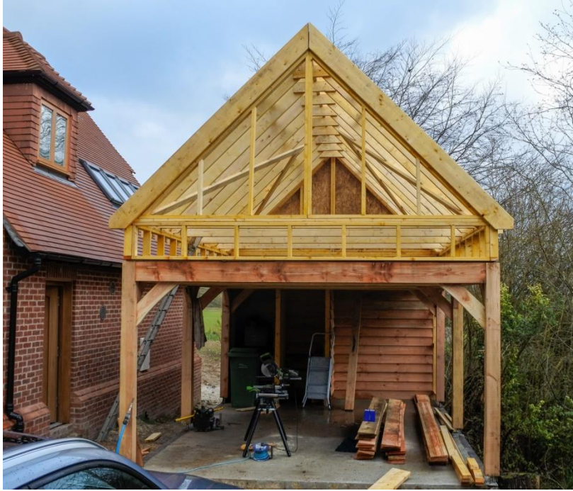
Figure 13. A dual use building with a garage below and bat roost above.
