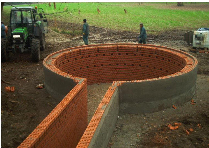
Figure 37. The Bulskampbeld hibernation site part way through construction building a brick dome on the chamber.
