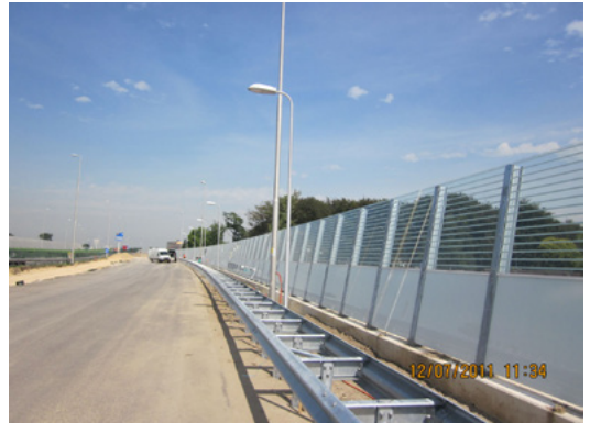
Figure 5.7. Partially shielded noise screens, installed during the construction of a new motorway in the Netherlands for avoiding light trespass to a compensation area with bat habitats (© V. LOEHR).
