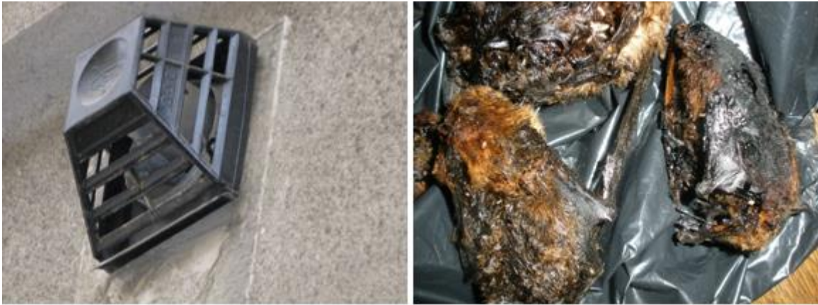
Fig. *. Noctules squeeze through horizontal fissures in metal protection and invade to gas heater and according the type they can be imprisoned here. Distress calls of bats often lure other bats. Once the heating season starts, bats are burned alive.
